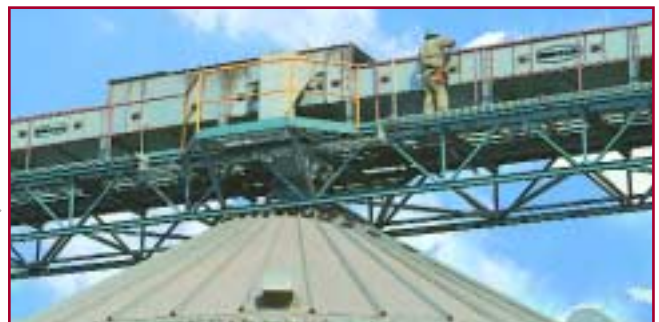
ENCLOSED ROLLER-BELT CONVEYORS
